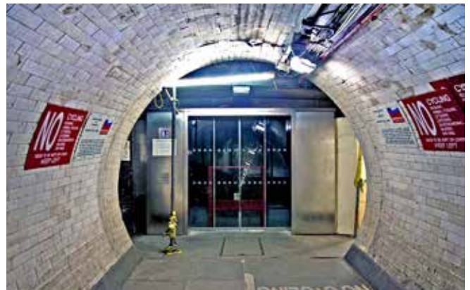
A new lift fitted at the north end of the Greenwich tunnel is not yet in use. The original wood panelled interior has been retained
